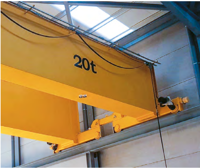
CRANE WITH DOUBLE END TRUCKS (EIGHT WHEELS)
